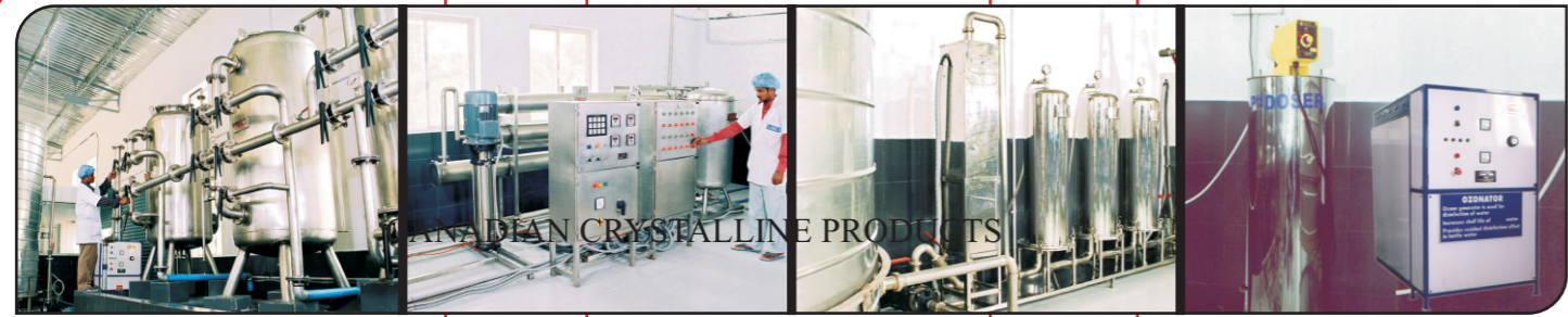
PRE FILTRATION SYSTEM
